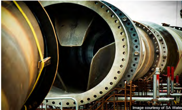
Figure 9.4. In-line static mixer at the Adelaide SWRO desalination plant prior to UF pretreatment. Approximate flow through this mixer is 6,250 m 3 /h.
