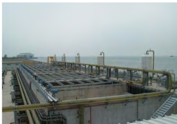
Figure 9.16. Dissolved air flotation and filtration (DAFF) installation at the Tuas, Singapore, SWRO desalination plant. Photo: PUB Singapore.
