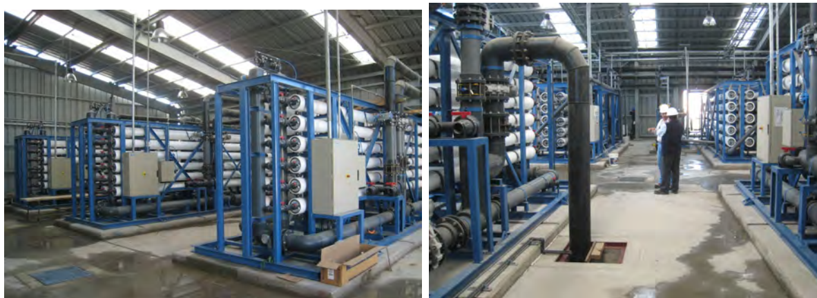
Figure 11.7.2. Ultrafiltration (left) and SWRO (right) trains at the Gas Atacama Plant.
