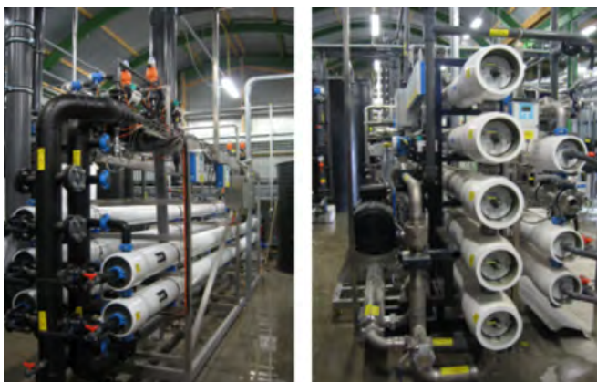
Figure 11.10.4. Demonstration plant ultrafiltration (left) and SWRO (the 5 pressure vessels on the left of the right hand image) and BWRO (the 3 pressure vessels on the right side of the skid).
