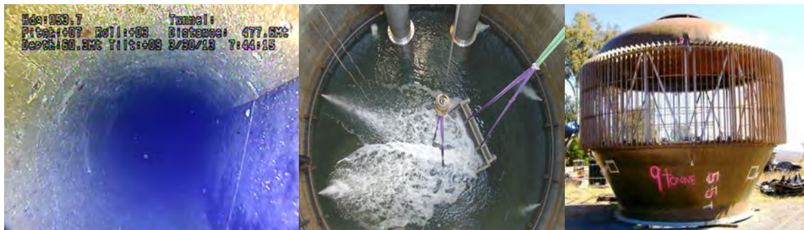
Figure 11.12.3. Intake tunnel (left), intake shaft with intake pumps (middle) and the intake coarse screen prior to installation (right).
