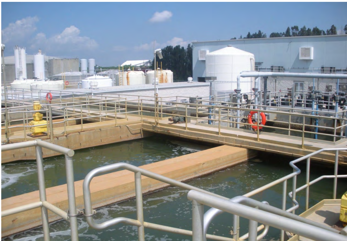
Figure 11.9.3. Normal pretreatment basin appearance (Voutchkov 2009).
