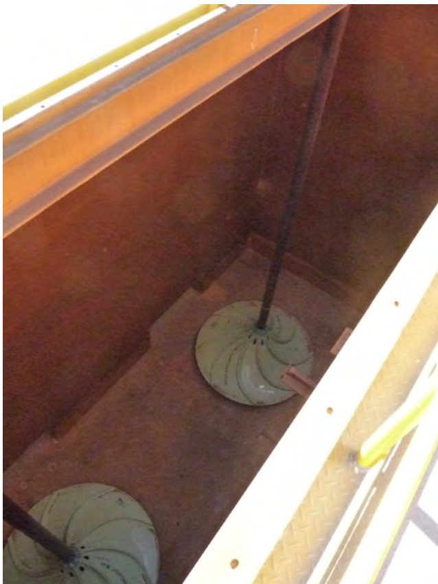
Figure 9.5. Flash mixers in a coagulation tank.
