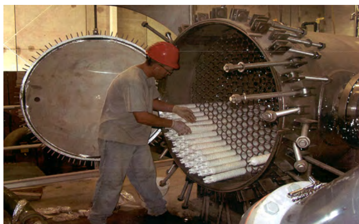
Figure 9.30. Cartridge filters installed in horizontal vessel.
